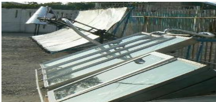
Fig. 1. General view of the experimental combined installation for producing hot water.
